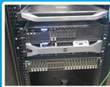
Active Directory Server Installation
